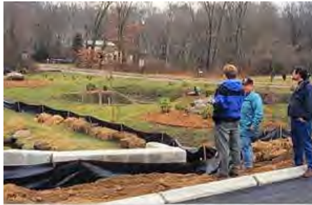
Construction reviewers periodically inspect construction sites to ensure that contractors have installed and maintained their erosion and sediment controls properly (Source: University of Connecticut Cooperative Extension System, 2000)
