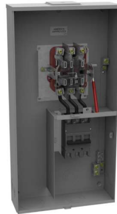
Figure 2 200-A Three-phase with Lever By-Pass
